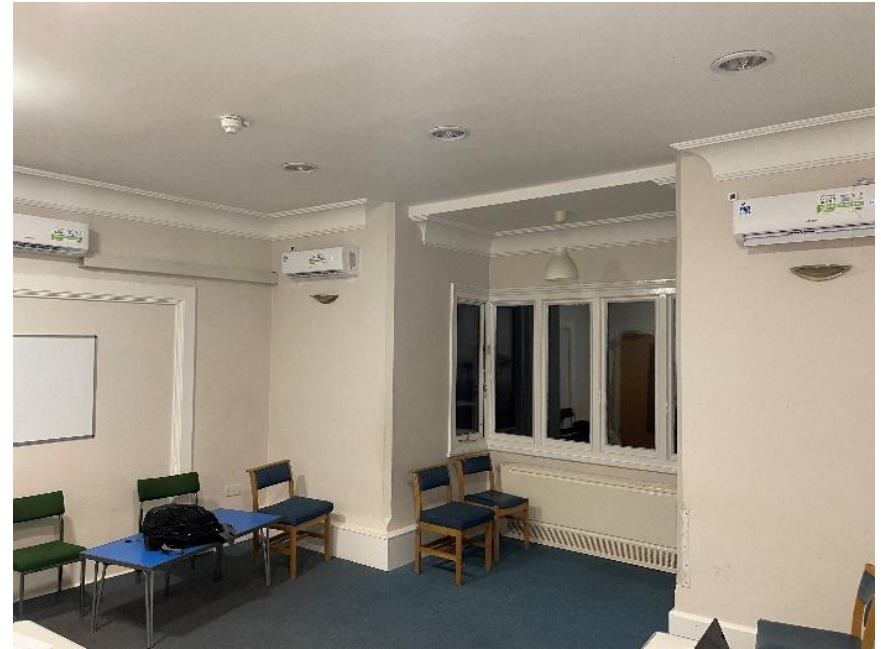
Air-to-air heat pump
